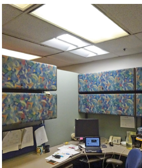
Lighting intervention. (top) An office worker uses a desktop luminaire; (bottom) CREE PoE SmartCast 2×2 troffers installed in an office workspace.
